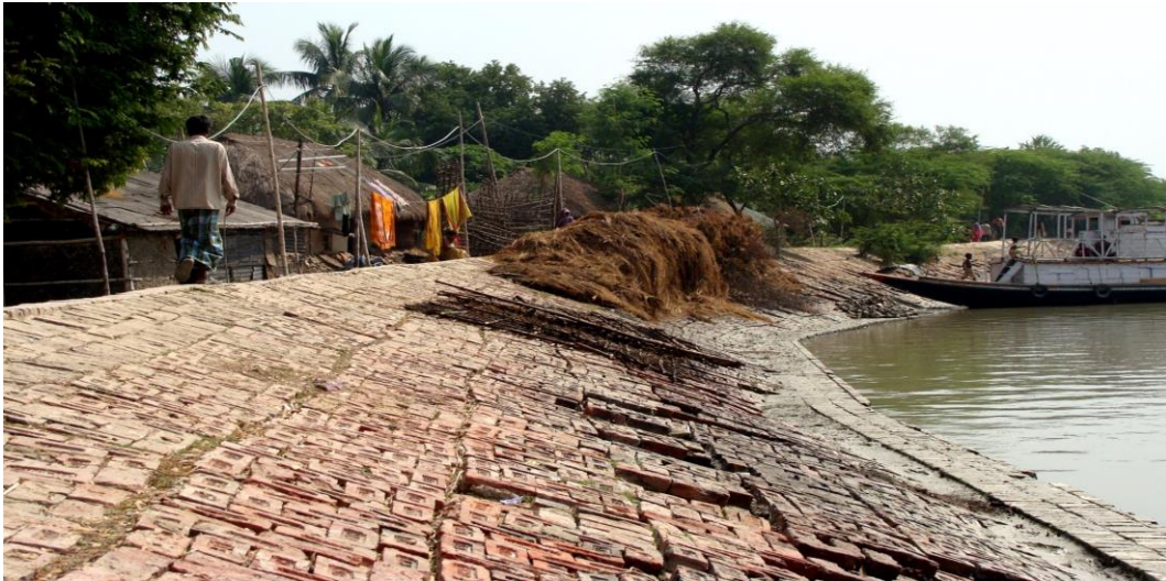
Fig. 3 Breaching of Earthen-Brick Embankment in the Indian Sundarbans leads to saline water intrusion
